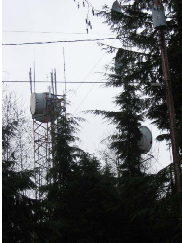
Figure 18. Communications infrastructure and power supply with no setback to forest vegetation.
